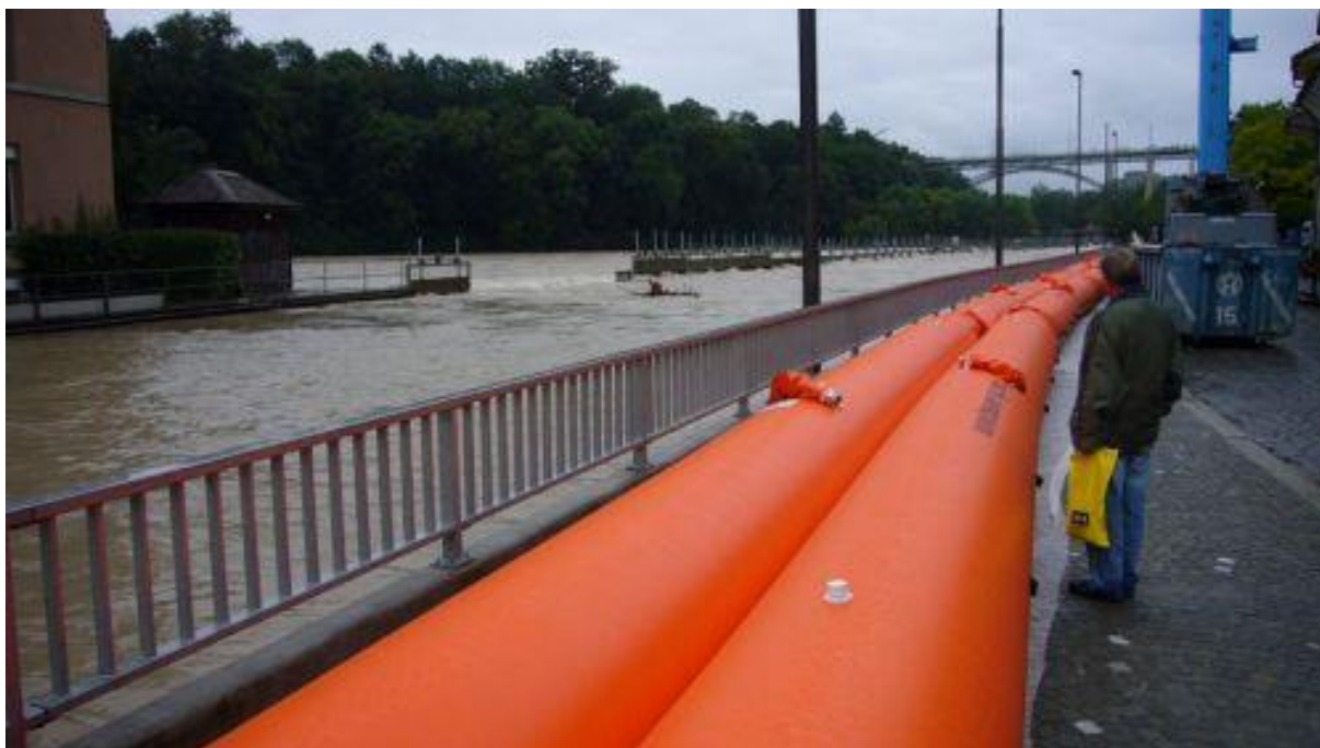
Figure 7: Beaver tubes as a mobile measure of intervention in the quarter of the “Matte” in the city of Berne © Professional fire brigade of the city of Berne, 2007
